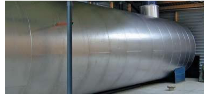
Horizontal/Plug flow digester
