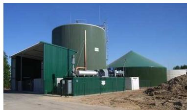
Energy Crop Biogas Plant
