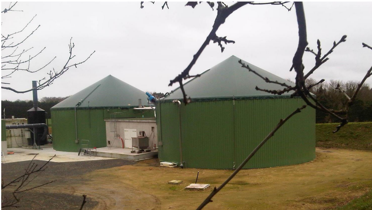
Secondary Digester B401 1.060 m 3
