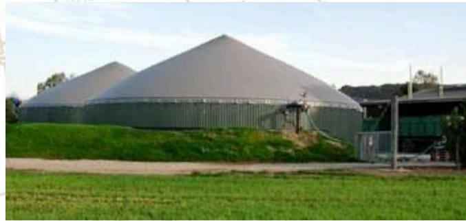
Flat digester with gasholder roof
