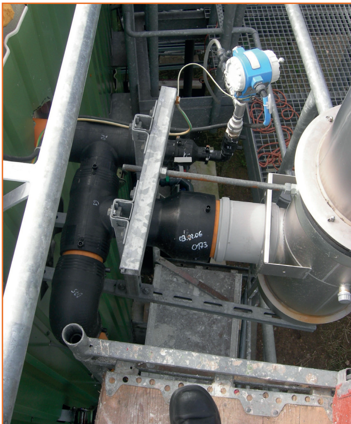
Figure 4: showing the overpressure valve
