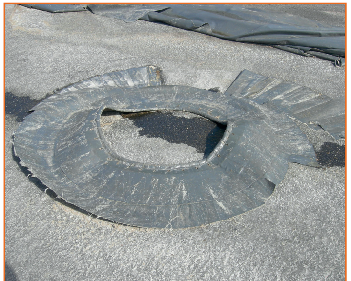
Figure 9: showing the holes causing the rupture
