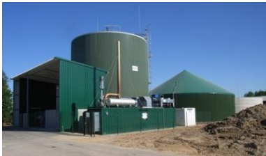
Energy Crop Biogas Plant
