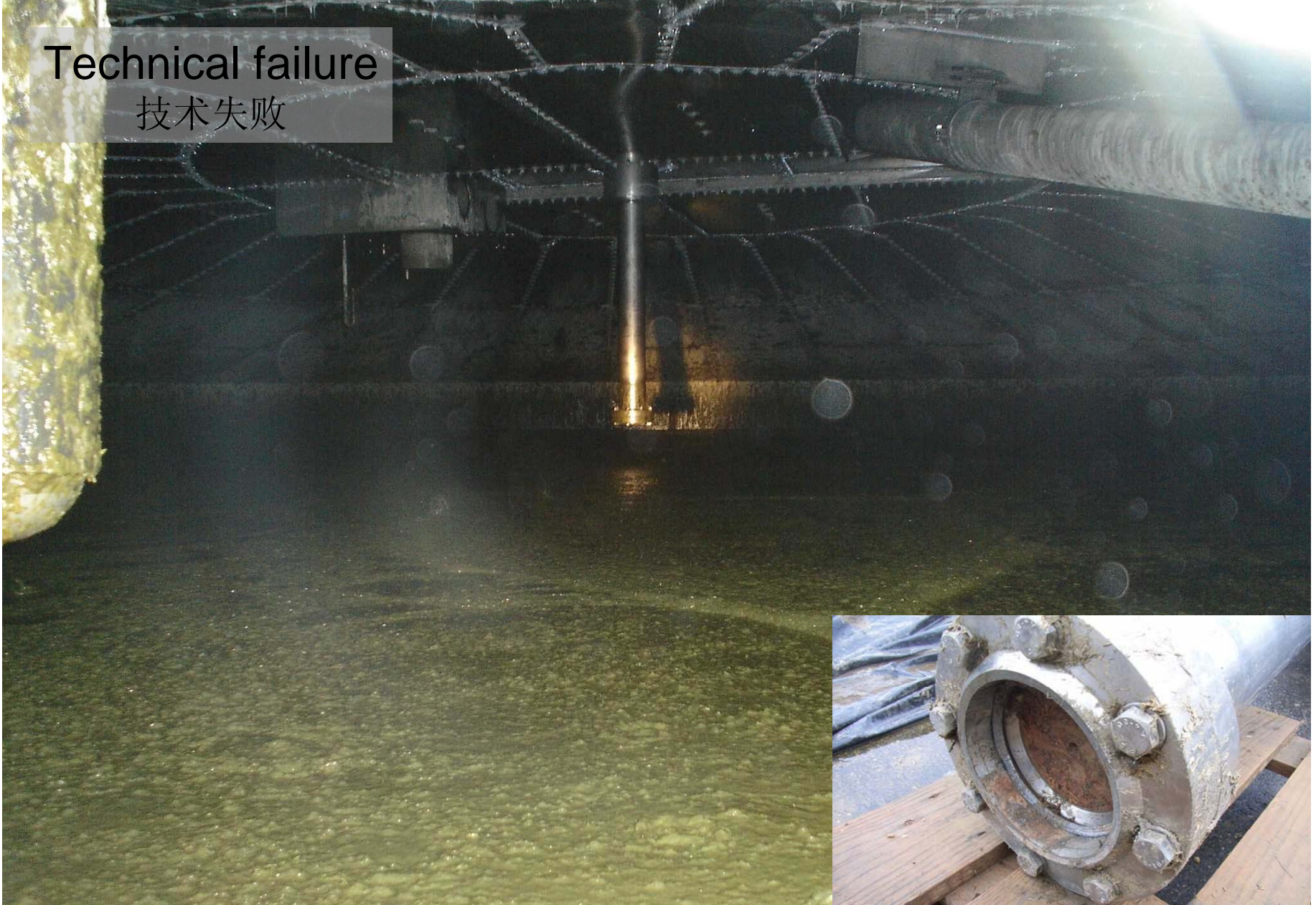
Broken shaft of the central stirrer 断轴中央搅拌器
