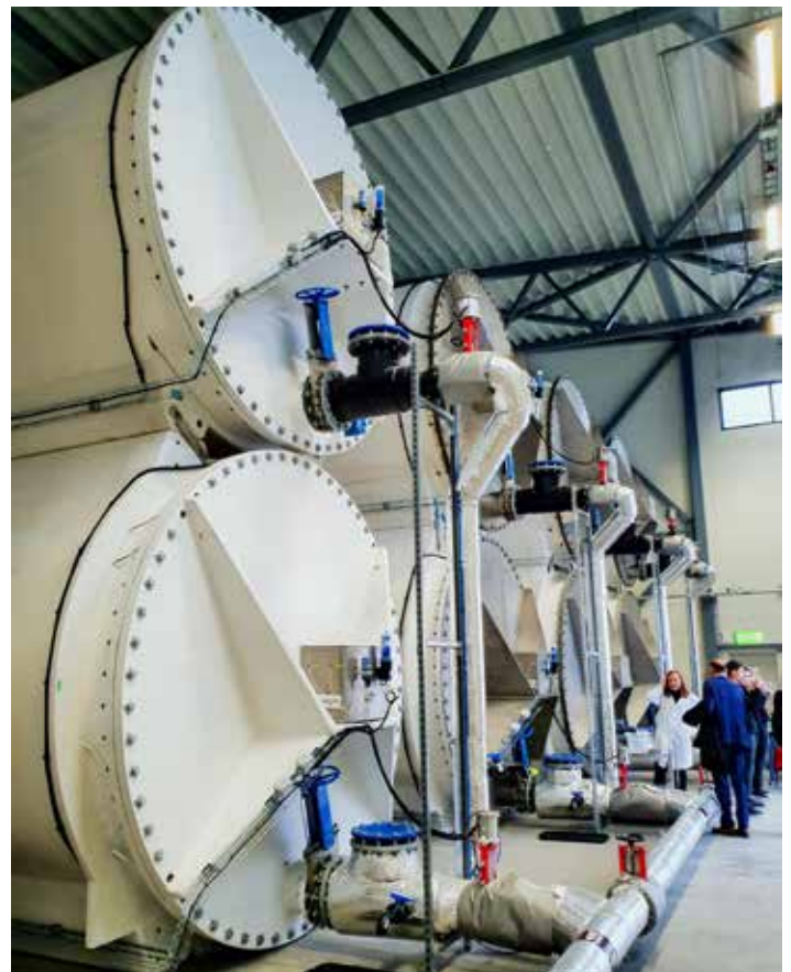
Stacked tanks showcases the company's scalability and design
